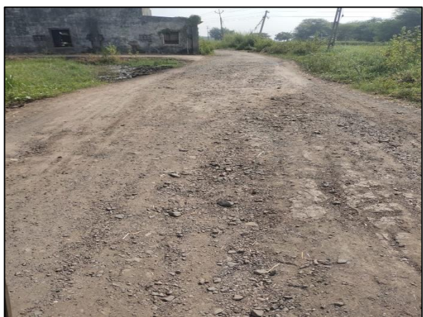
Fig 12.14 Road Condition of Ambheta
