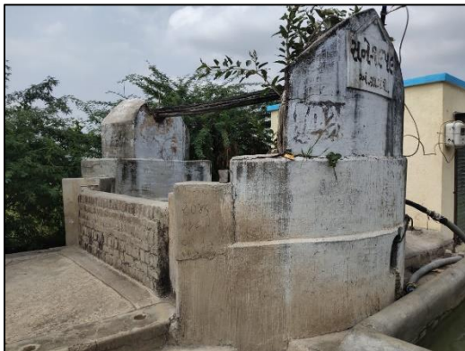
Fig.4.3 Under Ground Sump
